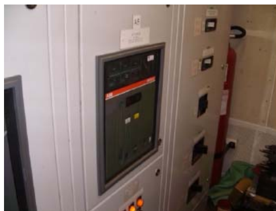
Switchboard crane breaker
