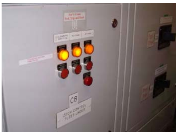
Switchboard open/reset command buttons
